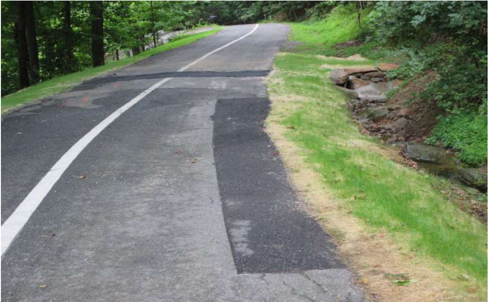
Wild Dogwood Trail: Finished Project (Maintaining our infrastructure) Replaced deteriorated culvert, note ditch work on left and right
