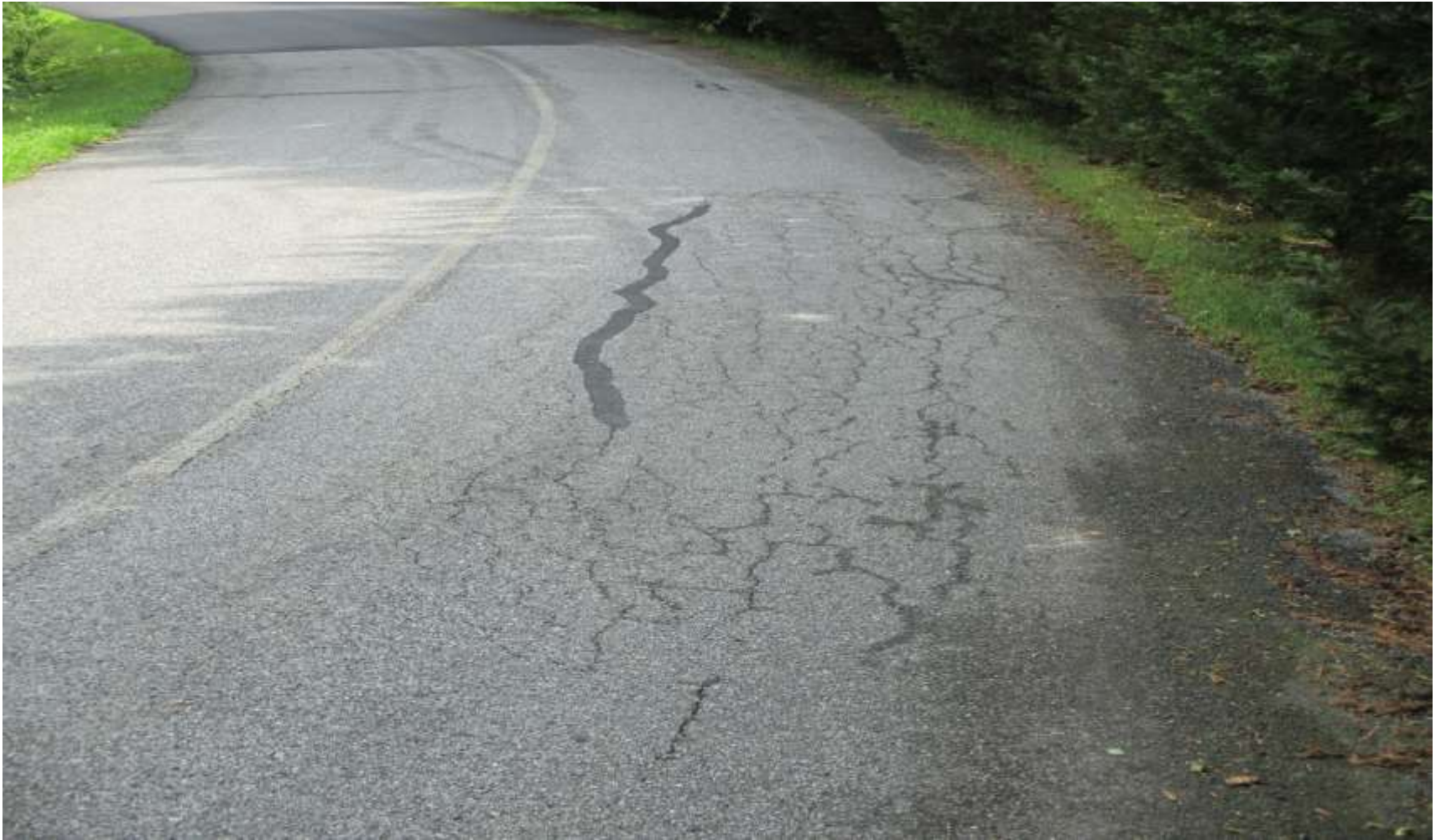
Vista Falls; new area of “alligatoring” developed since crack fill last fall
