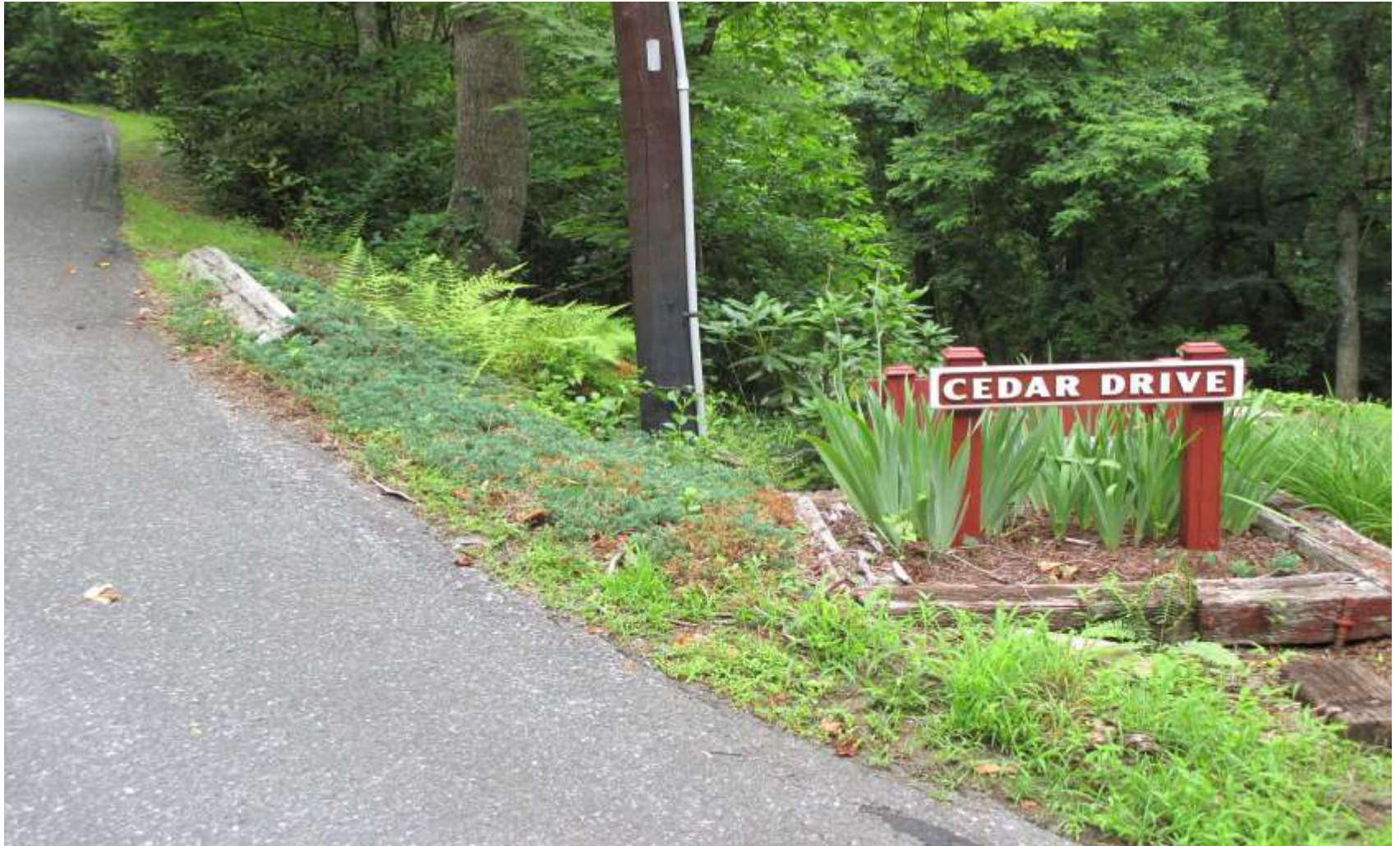
Cedar Drive Sign Box at Red Oak: Timbers are rotted, the slope is unstable and settlement will take the road with it
