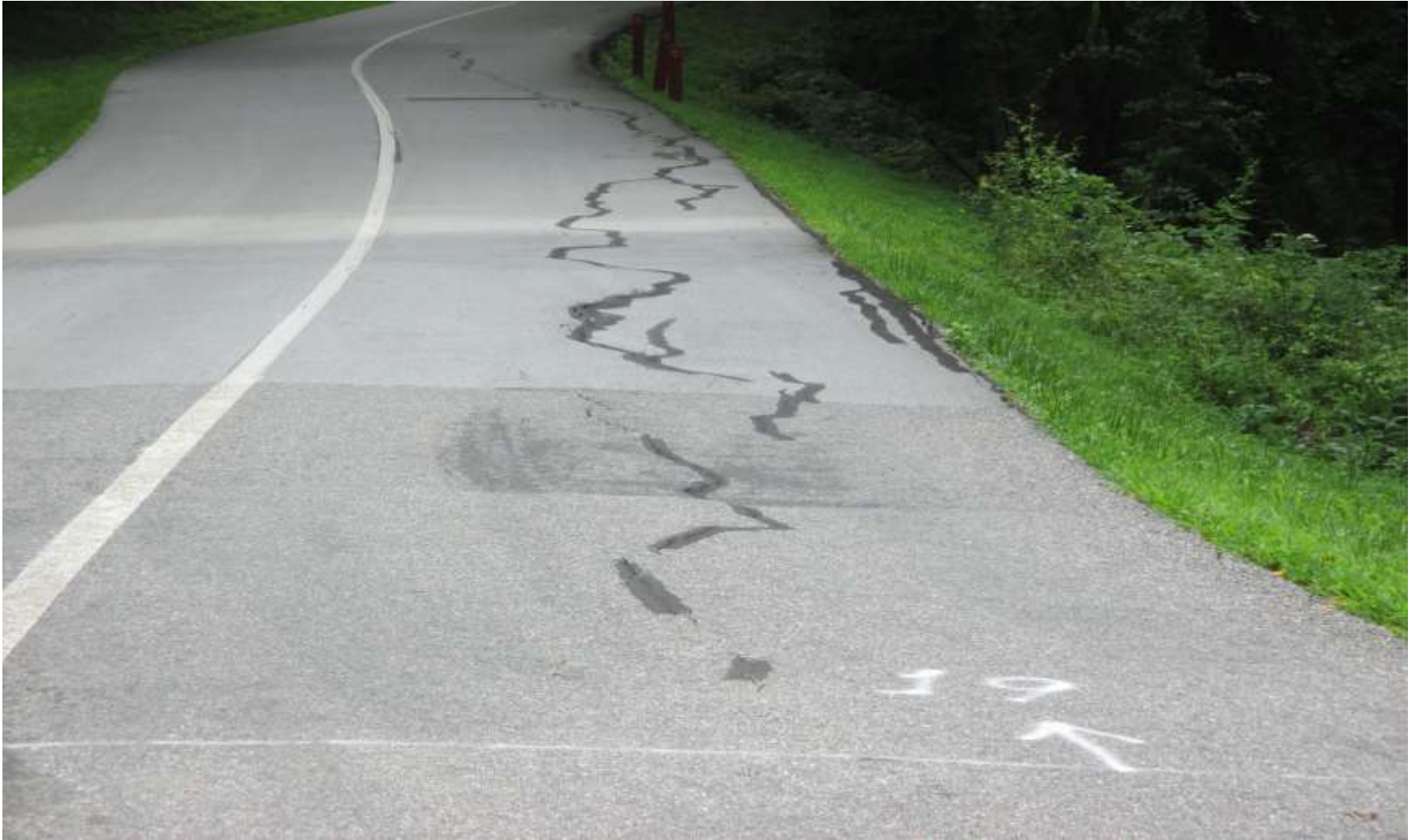
High Vista Drive at the Honey Locust stop sign, “Wedge” Repair required to shed water to inside ditch ($28k)
